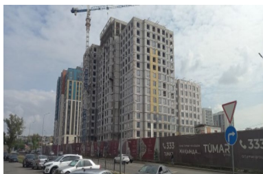
Photo 1. Failure of the urban planning to comply with the DPP and the construction site
