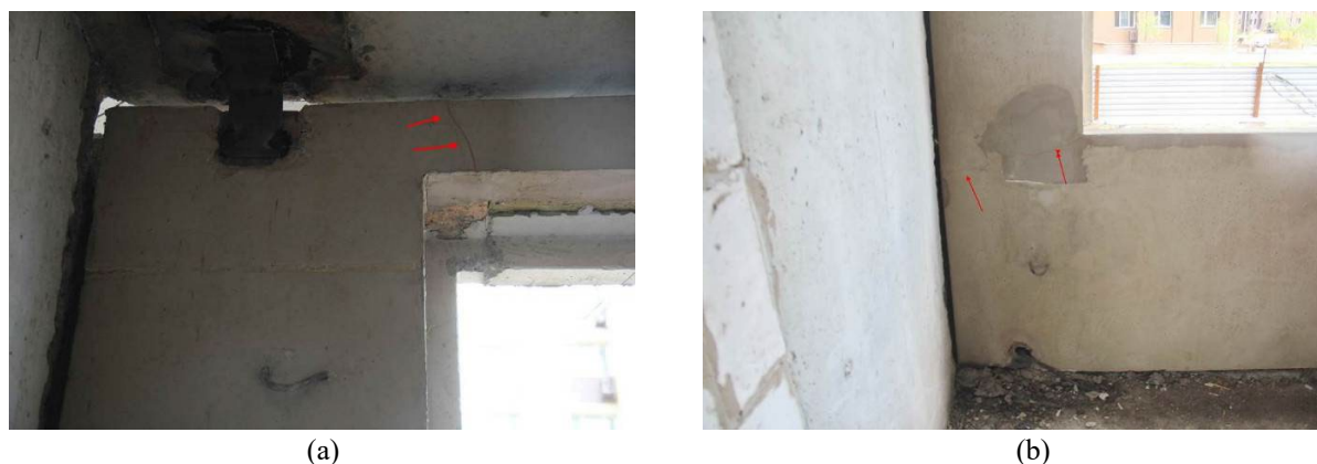
Figure 1 – Crack in the internal concrete layer of three-layer wall panels: a) crack at the top level of the wall panel; b) crack at the bottom level of the wall panel (Nuguzhinov et al., 2023).
