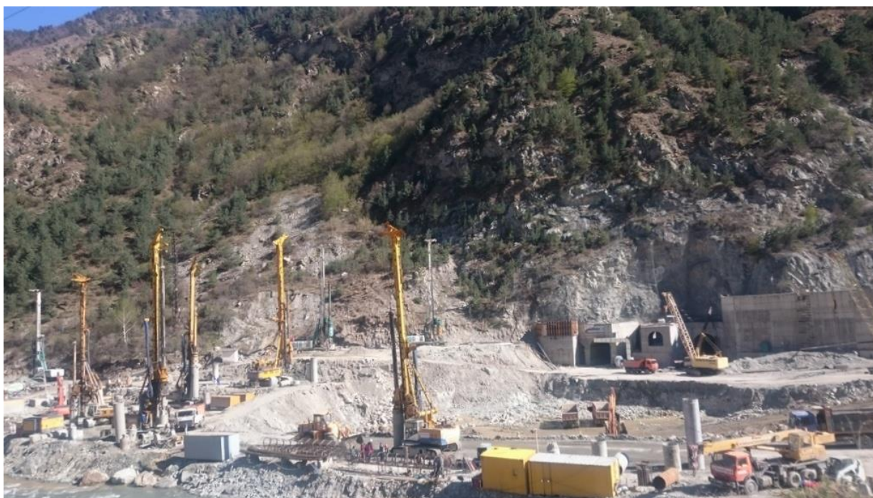
Figure 1 – Installation of secant drilled piles to protect the excavation of the Zaramagskaya HPP-1 building https://osetia.rushydro.ru/hpp/zaramagskaya-ges-1/
