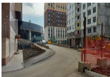
Photo 17. The incline leading from the main thoroughfare is angled towards the perimeter of the housing development
