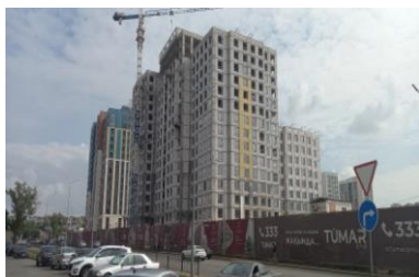
Photo 1. Failure of the urban planning to comply with the DPP and the construction site
