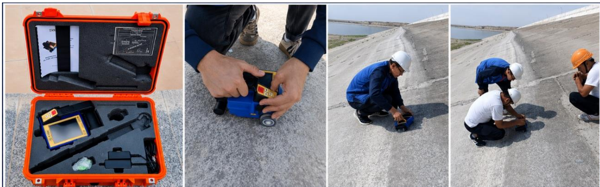
Figure 3 - Field application of the CK-1700 3D ultrasonic tomography system during inspection of concrete structures at the Tasotkel Reservoir emergency spillway (authors' material)
