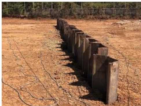
Figure 1 - Experimental installation of a steel vibration barrier for limiting wave propagation in the soil mass (author's material)
