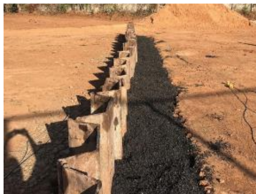
Figure 2 - Field installation view of a vibration-isolation trench barrier filled with a rubber-soil composite mixture(author's material)
