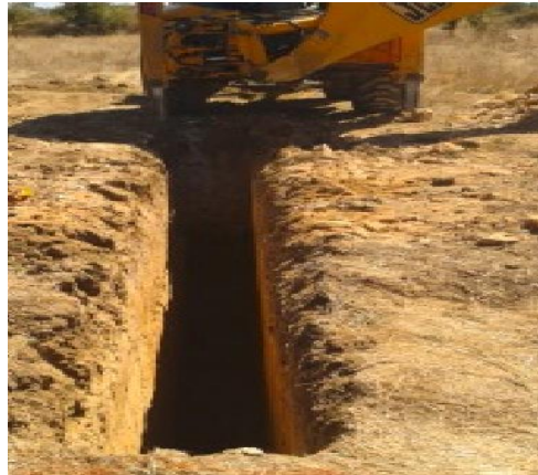
Figure 4 - Mechanized excavation process of a trench designed to limit the propagation of vibration waves (author's material)
