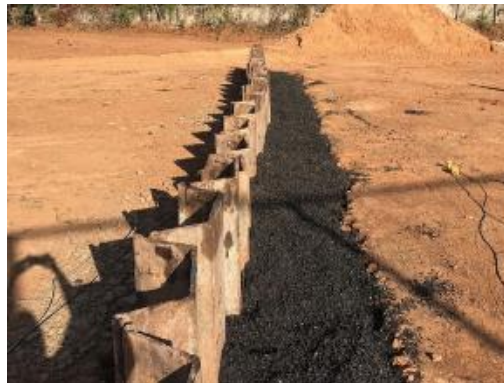
Figure 2 - Field installation view of a vibration-isolation trench barrier filled with a rubber-soil composite mixture (author's material)
