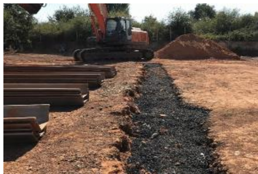
Figure 3 - Construction stage of the installation of a trench barrier designed to attenuate railway-induced Vibrations (author's material)
