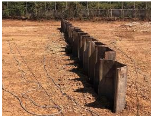
Figure 1 - Experimental installation of a steel vibration barrier for limiting wave propagation in the soil mass (author's material)
