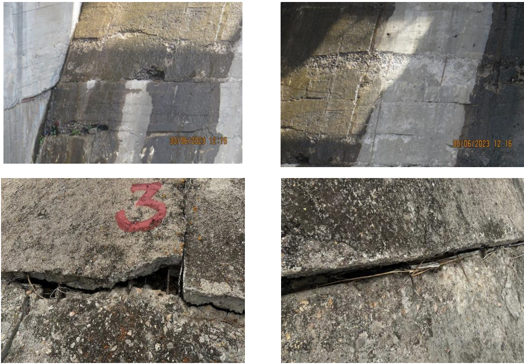
Figure 2 – Inspection fragments showing cracking and opening of joints in the deteriorated area. (author’s materials)
