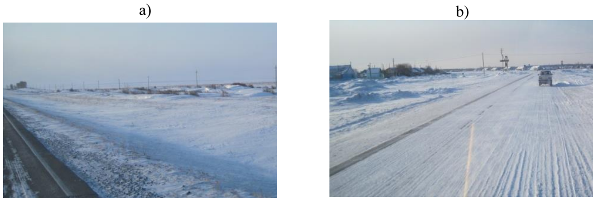
Figure 4 – Snow and ice formations on the pavement surface of the Kostanay-Surgan highway a – snow cover, section km 40–82; b – snow pack, section km 89–103 (author's materials)
