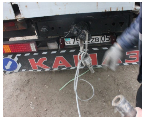
Figure 6 - Insertion of a cable connection with a power plant (car) (author's materials)
