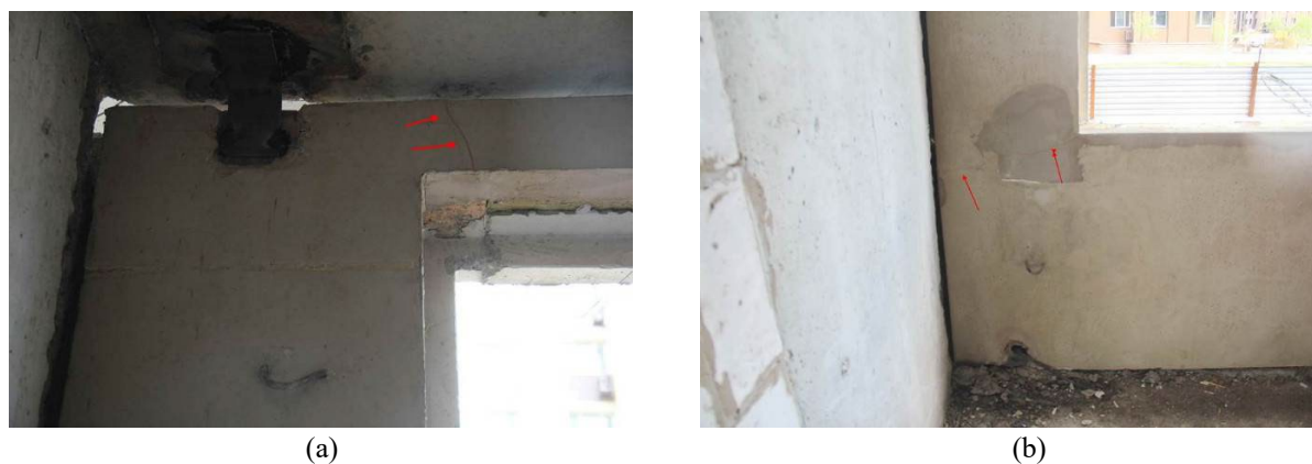
Figure 1 – Crack in the internal concrete layer of three-layer wall panels: a) crack at the top level of the wall panel; b) crack at the bottom level of the wall panel (Nuguzhinov et al., 2023).
